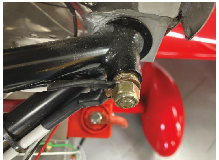
This engine mount bolt has been used as a grounding point, leaving too few threads protruding beyond the nut. For many reasons, an alternate ground point should have been used.
