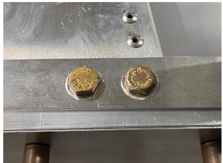
The score marks around these bolt heads were caused by rotating the bolt with a socket wrench. Such damage can be avoided by rotating the nut, not the bolt.
